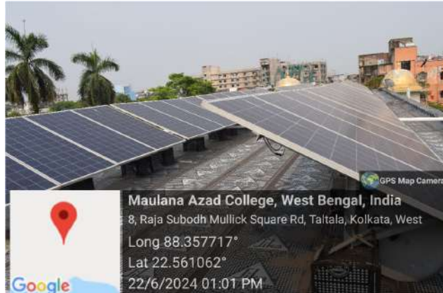
Rooftop Solar Panel
